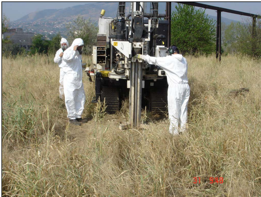
Figure 2: Soil drilling at the dumpsite of alpha and beta isomers of HCH
